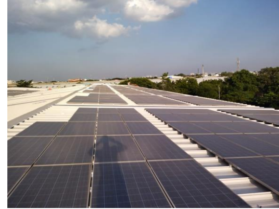
200 kWp Solar PV Rooftop Solar at Warehouse
